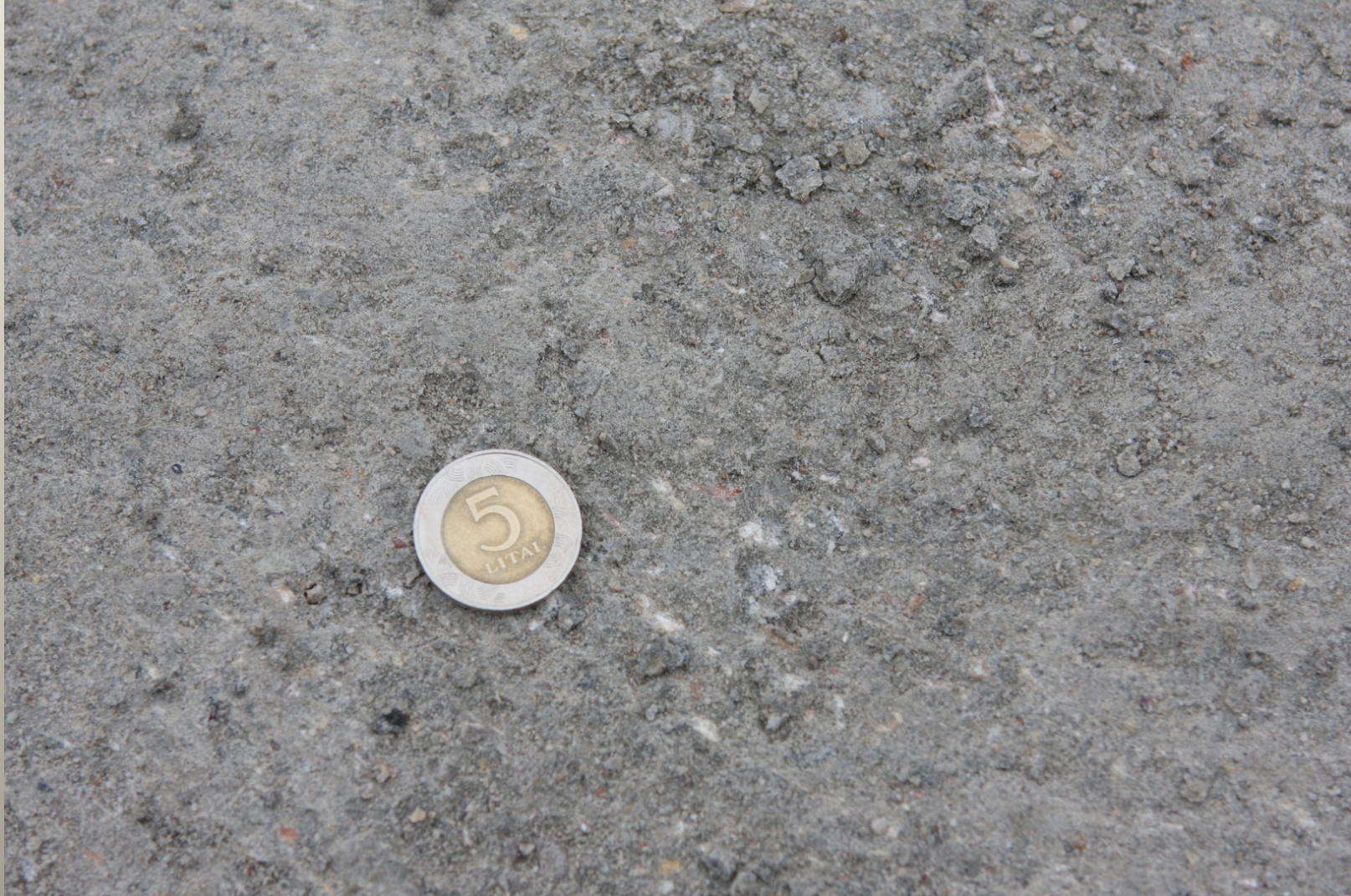
Typical damages of concrete surface after freeze-thaw cycles, deicing salt, and harsh car's traffic.
