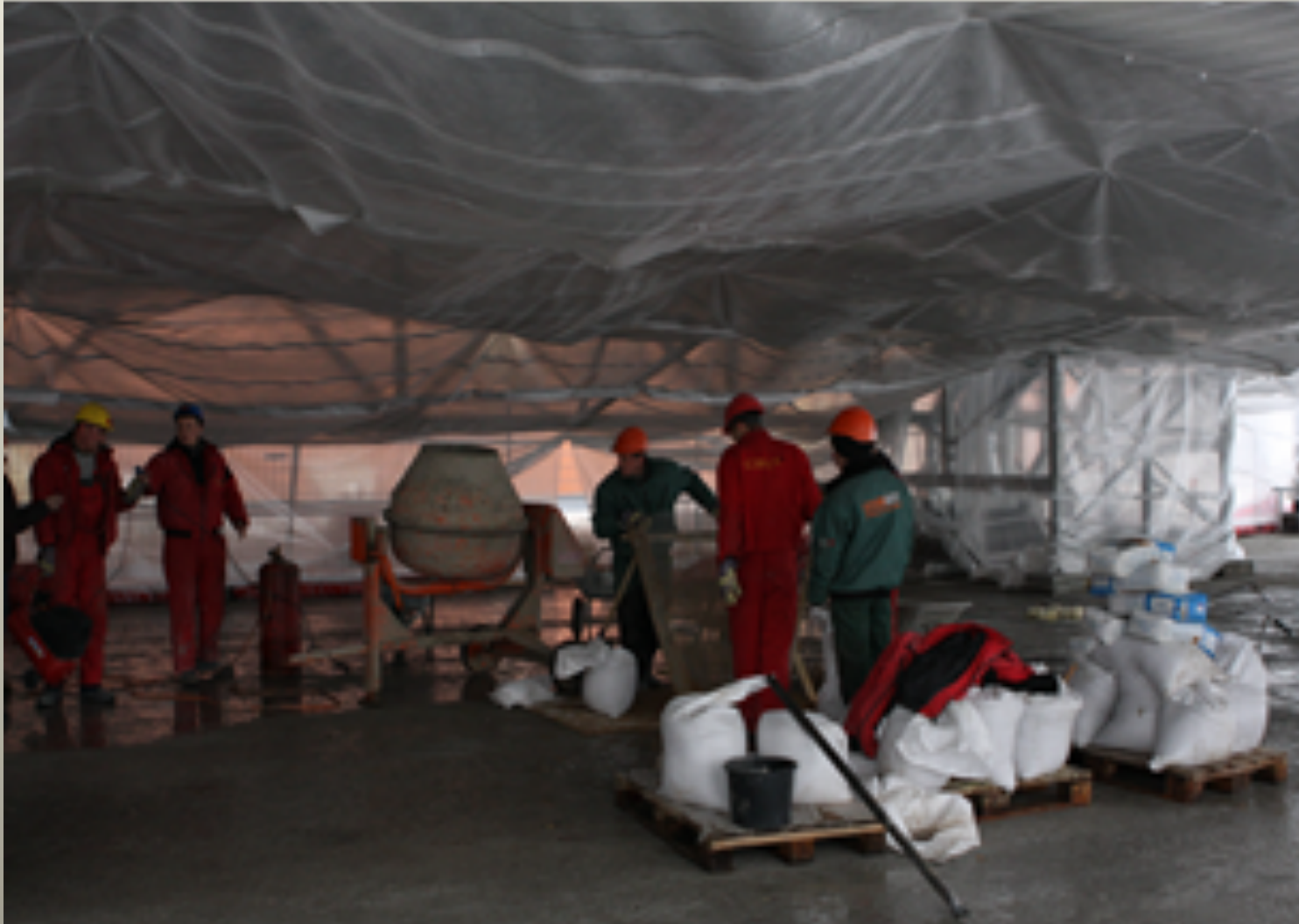
PLASTCRETE preparation by dry mixing of Kalmatron® KF-A, local sand and cement just on a job site.
