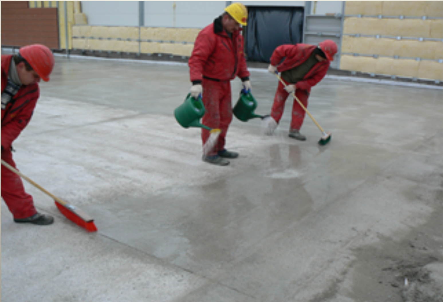
Distribution of diluted KF-G by the brushes for economical distribution by 2 Liters/m 2 .
