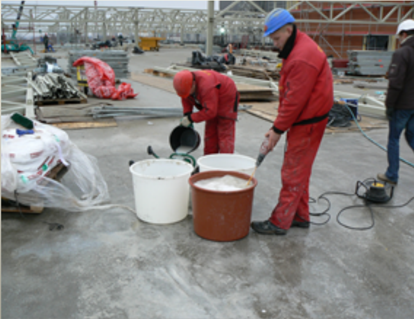
Kalmatron® KF-G preparation by dilution of its 300 Grams by 1 Liter of water to provide chemical type of adhesion of damaged and contaminated concrete with PLATSRCRETE layer.
